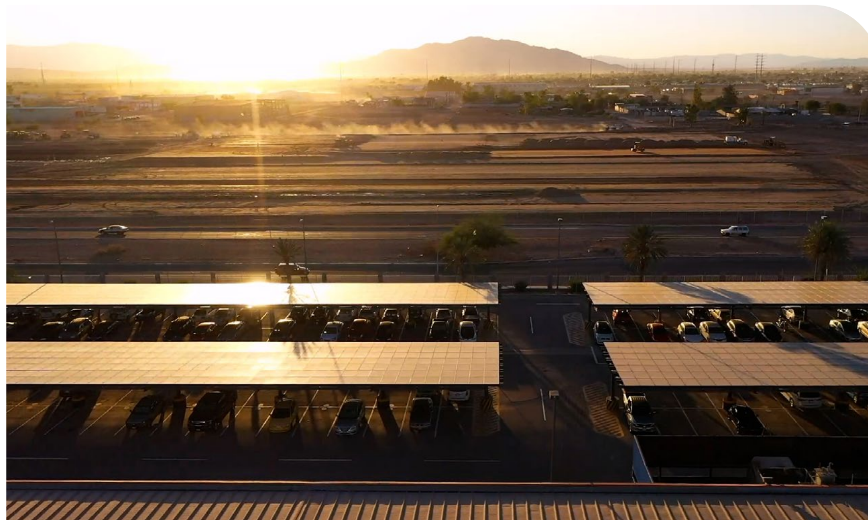
Carport solar in Mexicali, Mexico facility
