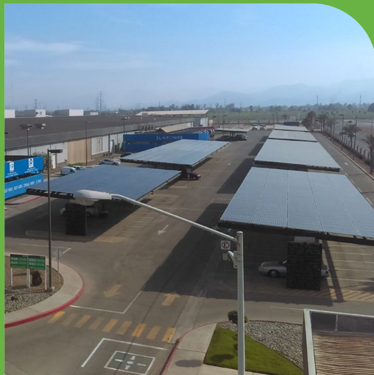
Solar panels installed as part of our carport project in our Mexicali plant (SPMX1)
