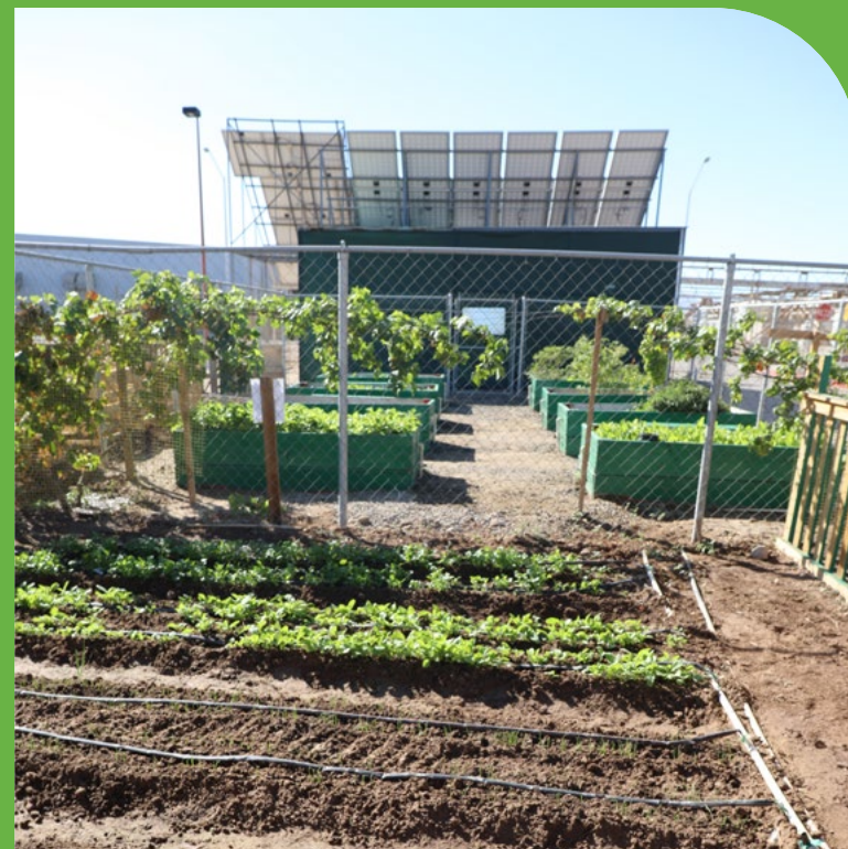
Solar panels installed atop our organic garden
