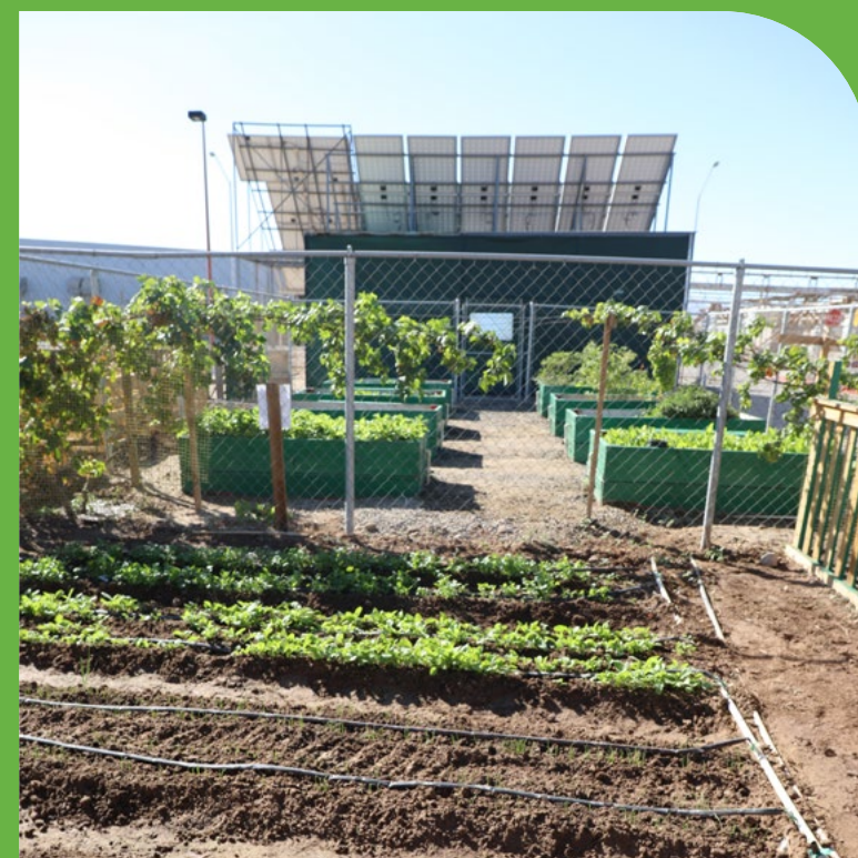
Solar panels installed atop our organic garden
