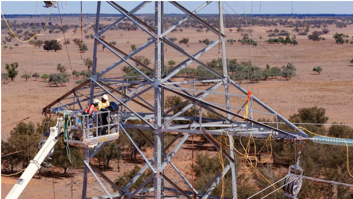
Construction of the Energy Connect transmission line is paving the way for renewable energy developments. (Supplied: Elecnor Australia)
