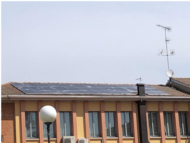
A PV system damaged by the hail storm that hit northern Italy on July 23. Image: Leonardo Setti
